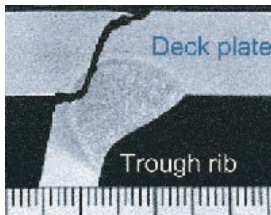
図 デッキプレート貫通型き裂 (S.Ono, T.Shimozato, N.Inaba, and C.Miki : Wheel running fatigue test for orthotropic steel bridge decks, 58th IIW Annual Assembly, Doc.XIII-2070-05, 2005.)
